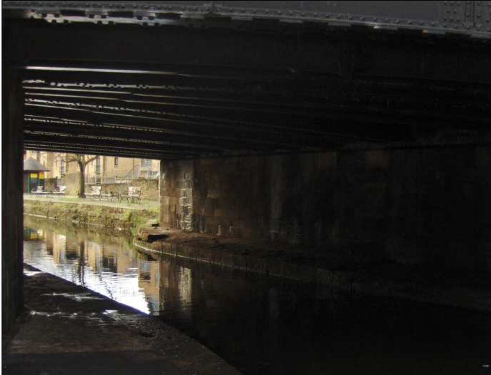
Photograph showing the darkness under the Penny Street Bridge
